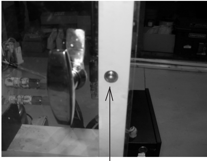
Figure 6. Safety Door Interlock
